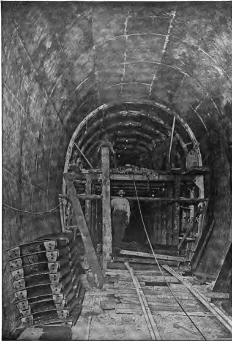
PLATE 107. —Contract 12. Blaw Grade Tunnel Forms. Form was filled in 30-foot lengths and collapsed by pulling in sides at mid-diameter with turnbuckles, unbolting ribs at center and lowering with jacks on wooden carriage running on rails. See also Plate 113.
